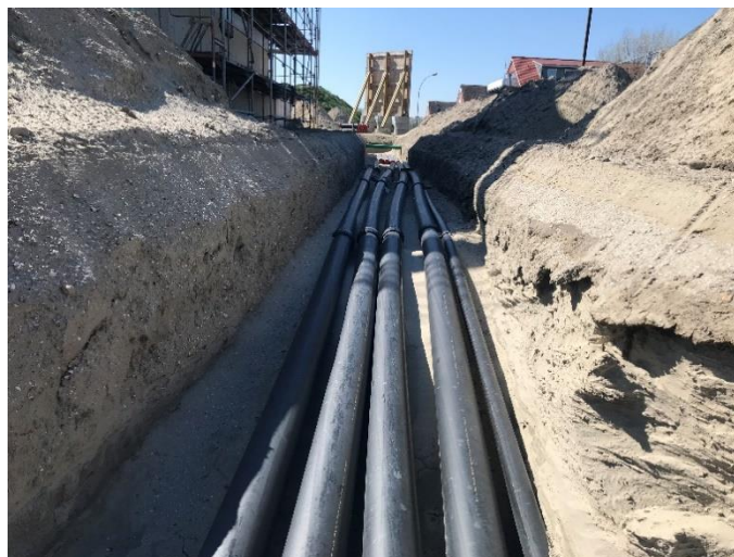
Figure 16 PE pipes for sea water
