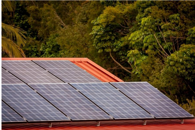
Figure 33 Arrays of solar panels on the roof of a house (public domain)
